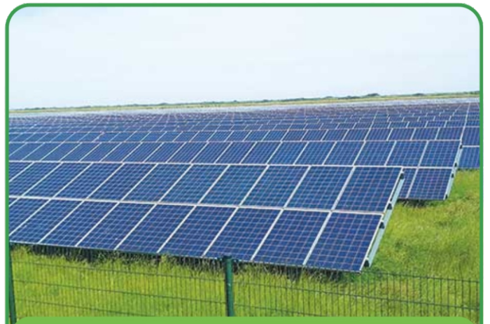
1.1 MW JHALERA, HIMACHAL PRADESH
