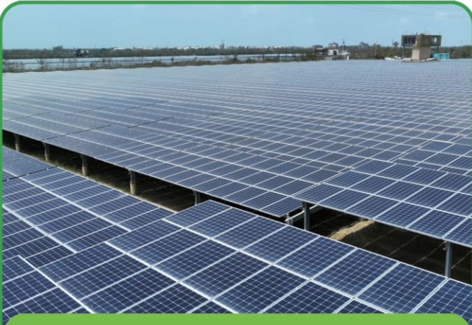
6 MW AT GUJARAT
