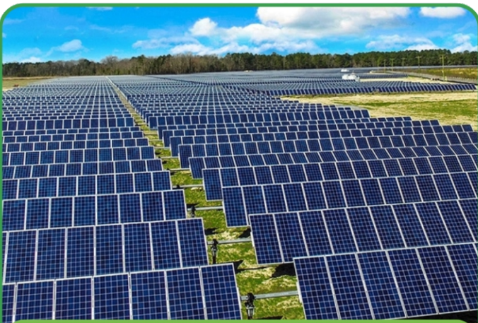
3 MW NAGORI, RAJASTHAN
